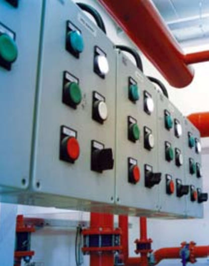
Manual/remote automatic control of fire extinguishing pumps.
