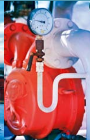
Detail of flow measuring equipment.
