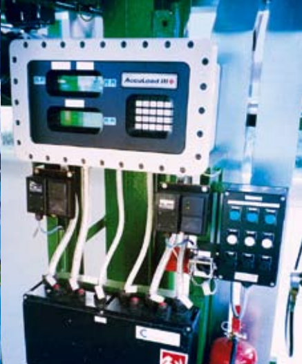
Accumul III, the batch controller, and ELBC2 card readers ensure the process level of automation.
